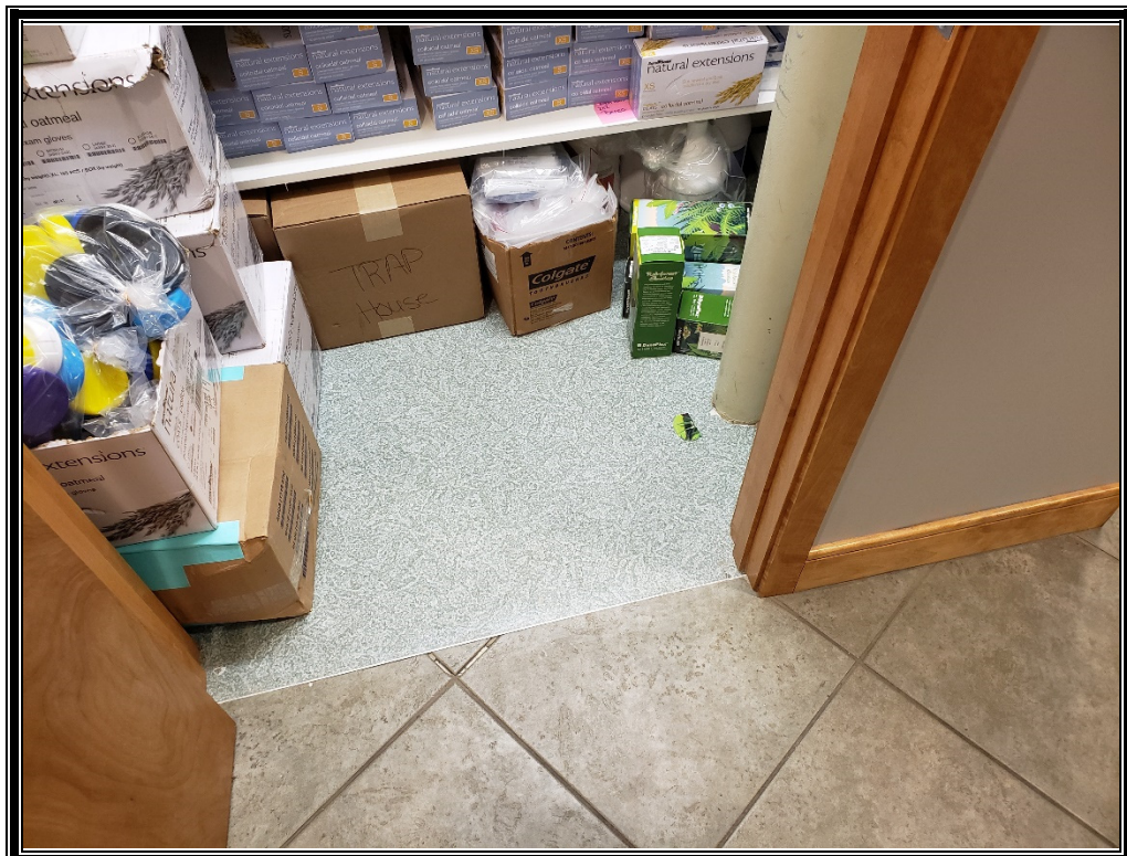
Photo 14: Viewing at sheet vinyl flooring in a closet of the Hickman Orthodontist unit.
