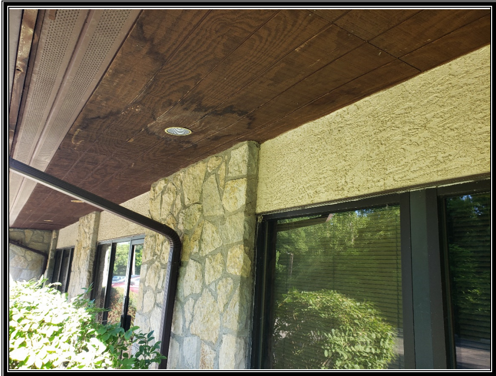
Photo 5: Viewing at the office building exterior materials including stucco, stone, window caulk, and wood trim.
