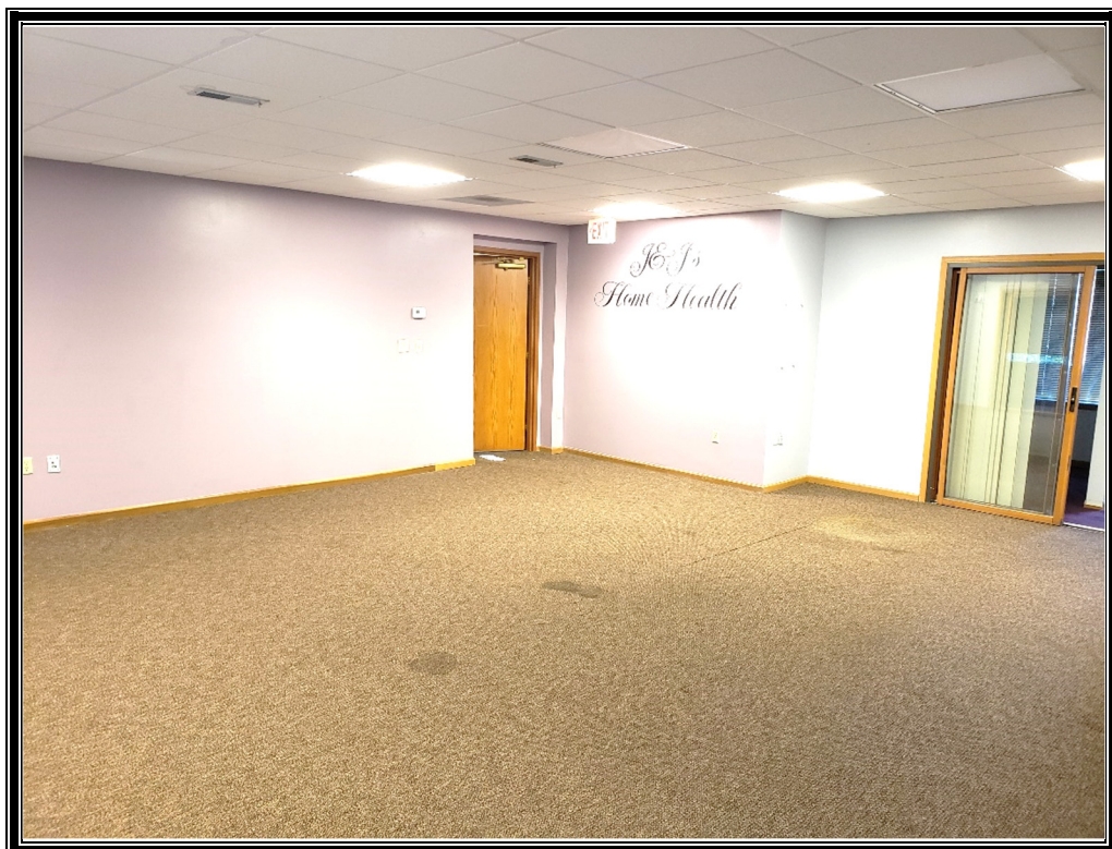
Photo 12: Viewing at the vacated J&J's Home Health unit with acoustical ceiling panels, drywall, and carpet.
