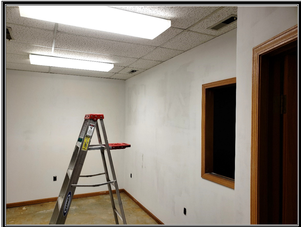
Photo 7: Viewing at acoustical ceiling panels, drywall, and exposed carpet mastic in Unit 201.
