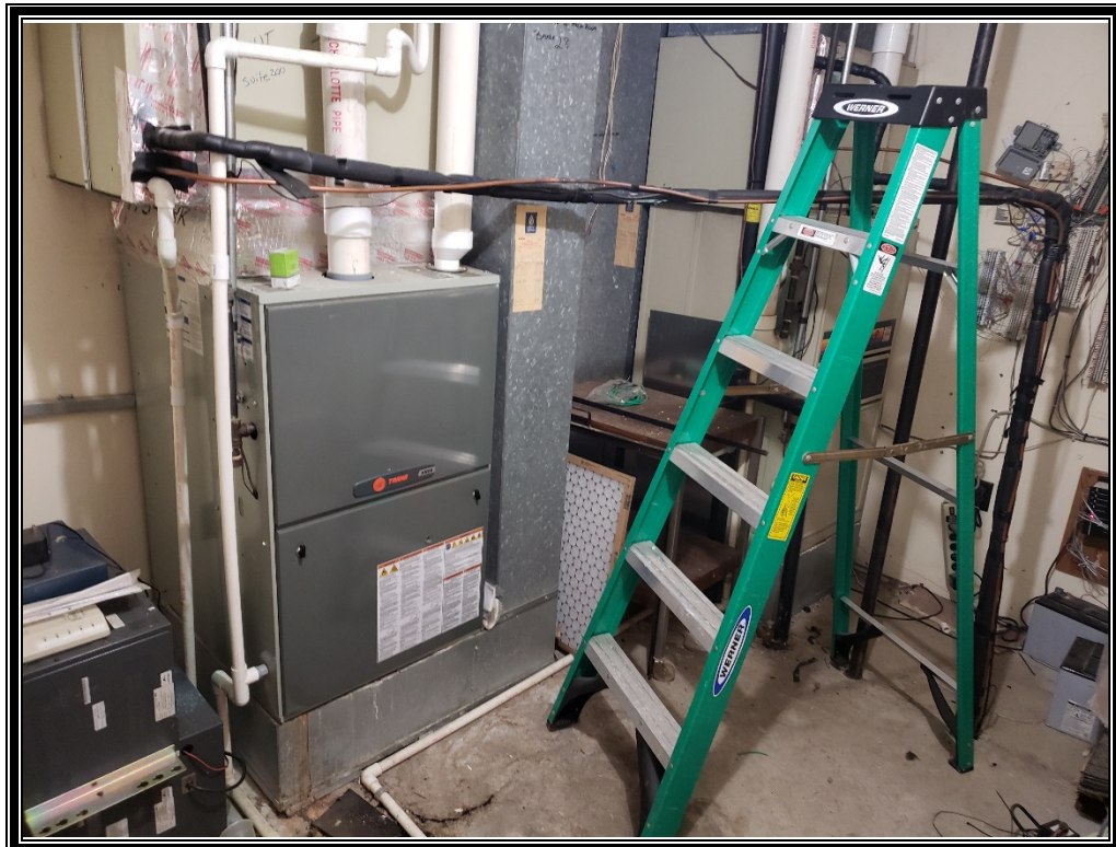
Photo 11: Viewing at one of the natural gas forced air furnaces in the building.
