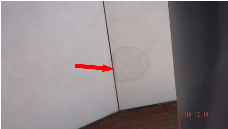
4c. Staining on plaster ceiling (see #4 on elevation photo for location).
