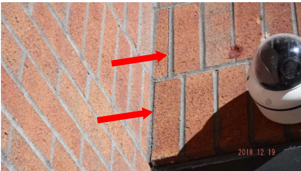
1b. Cracked/shrunk mortar joints (see #1 on elevation photo for location).
