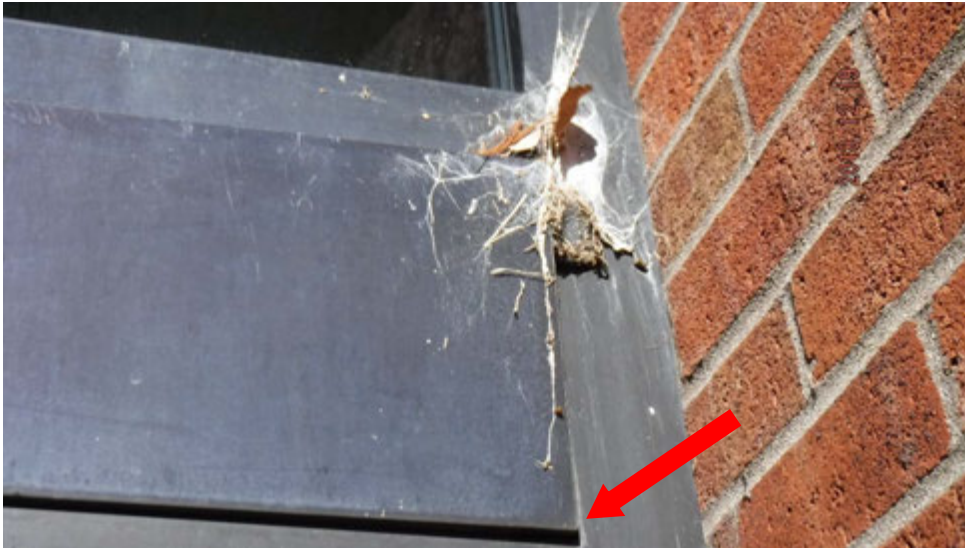
8c. Loose window trim metal between window sets. (see #8 on elevation photo for location).
