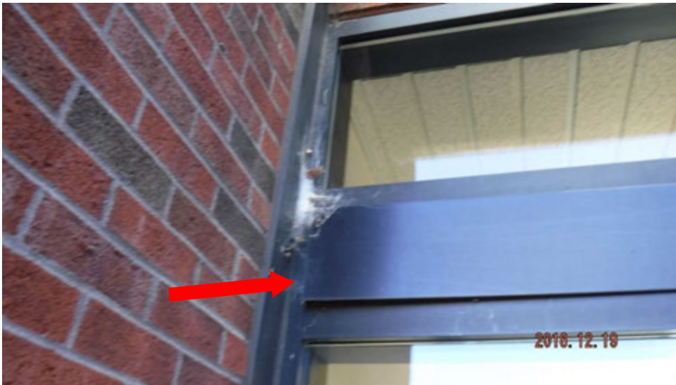
7a. Loose window trim metal between window sets (see #7 on elevation photo for location).
