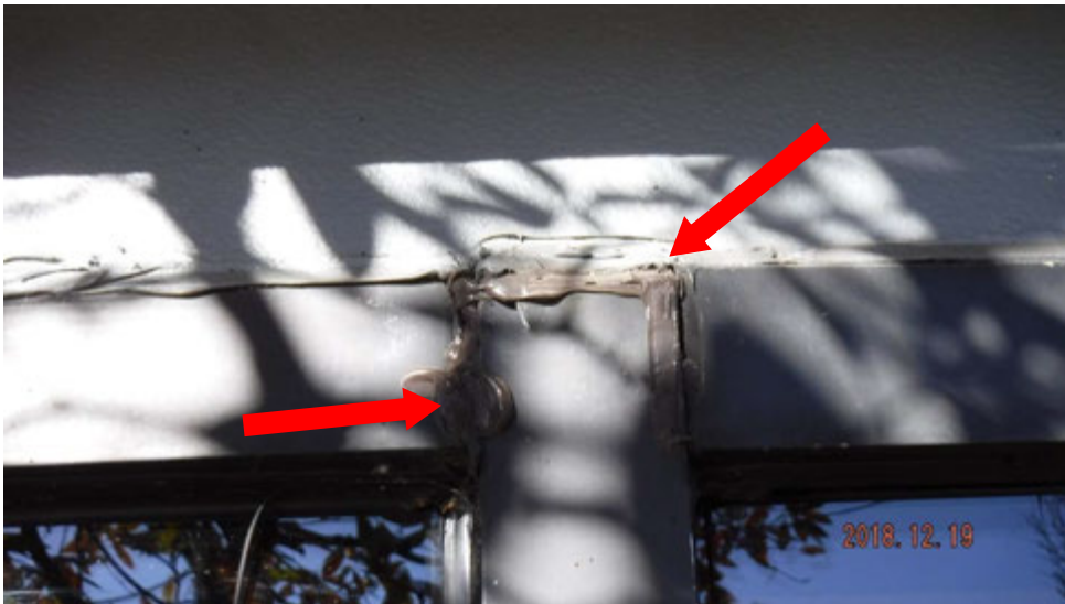
9c. Heavy top caulking over window frame/pressure plate joints (see #9 on elevation photo for location).
