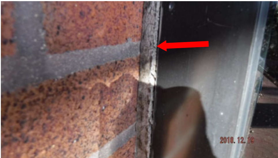
6d. Cracked/shrunken sealant joint (see #6 on elevation photo for typical locations).
