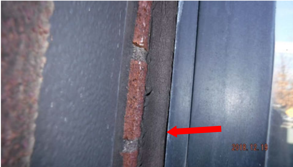
4a. Cracked/shrunk sealant joint (see #4 on elevation photo for typical locations).
