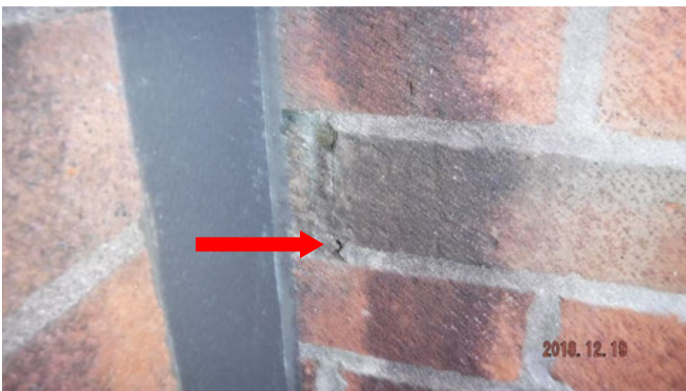
1b. Deteriorated mortar joints (see #1 on elevation photo for location).
