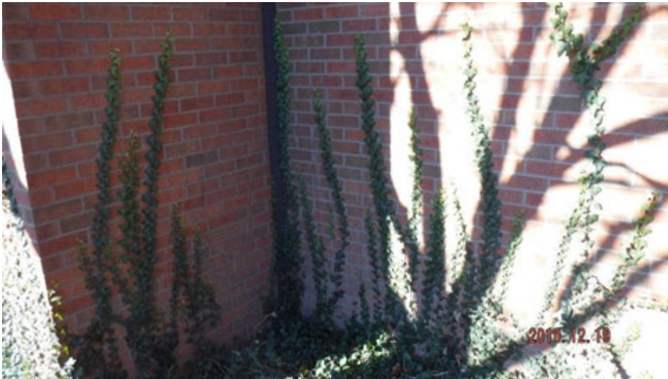
3a. Vegetation growth on walls (see #3 on elevation photo for typical location).
