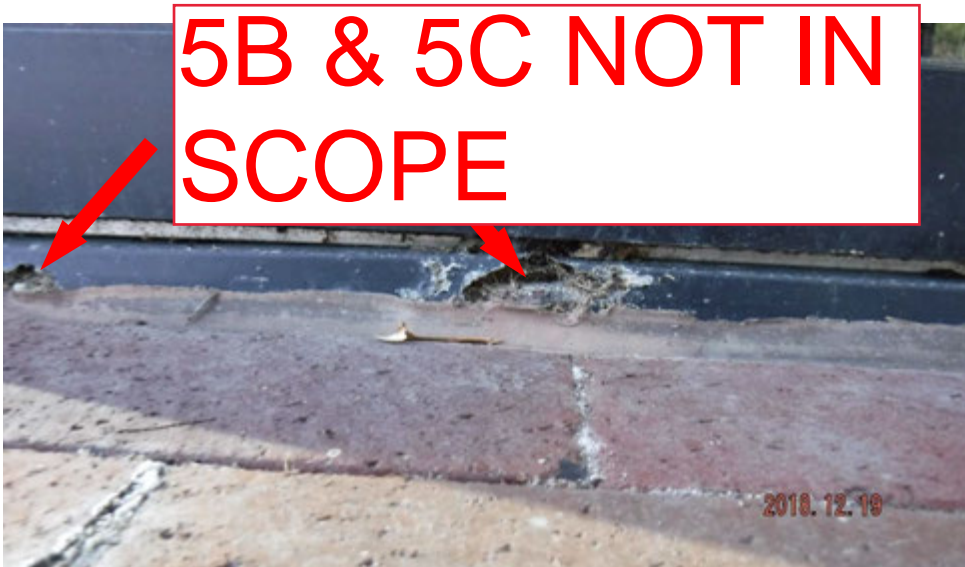
5c. Corroded steel member(s) at base of window where it sets at ground level (see #5 on elevation photo for location).
