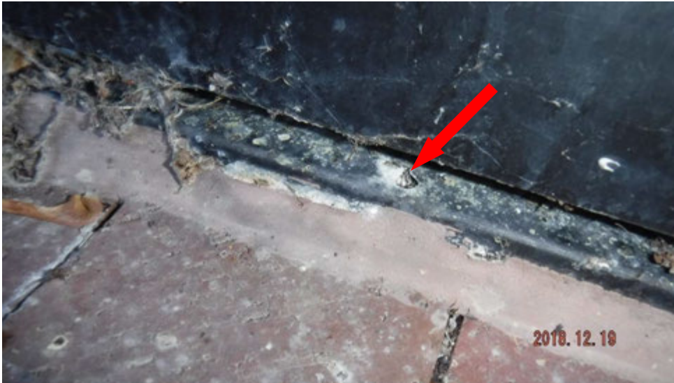
7b. Corroded steel member(s) at base of window where it sets at ground level (see #7 on elevation photo for location).
