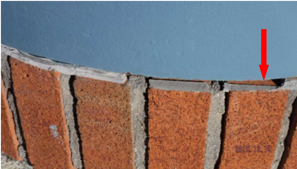
3a. Cracked/shrunk sealant joint (see #3 on elevation photo for location).
