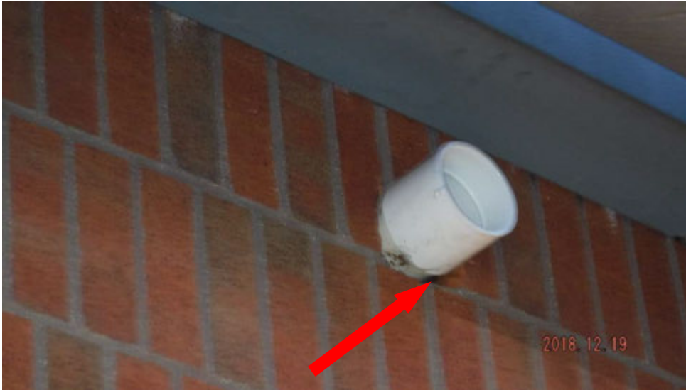
2a. Missing sealant joint (see #2 on elevation photo for typical location).
