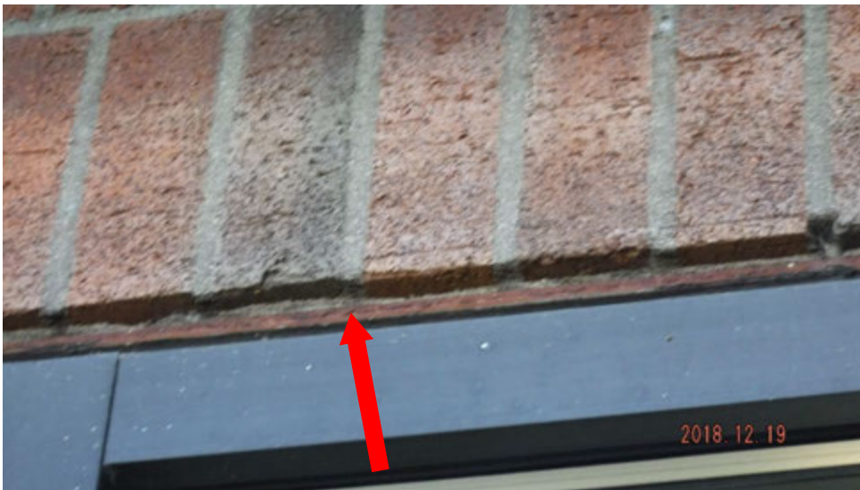
6b. Corrosion on window lintel (see #6 on elevation photo for typical locations).
