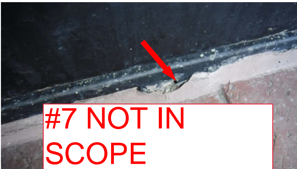
7a. Corroded steel member(s) at base of window where it sets at ground level (see #7 on elevation photo for location).
