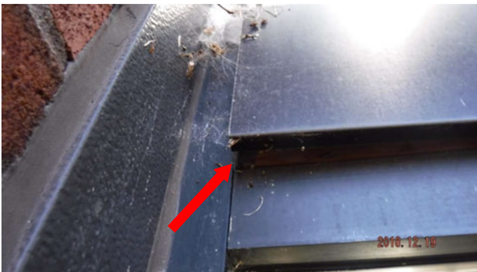
7b. Loose window trim metal between window sets. Wood could be observed behind the loose metal (see #7 on elevation photo for location).
