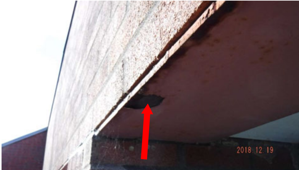
11a. Corrosion on window lintel (see #11 on elevation photo for typical locations).
