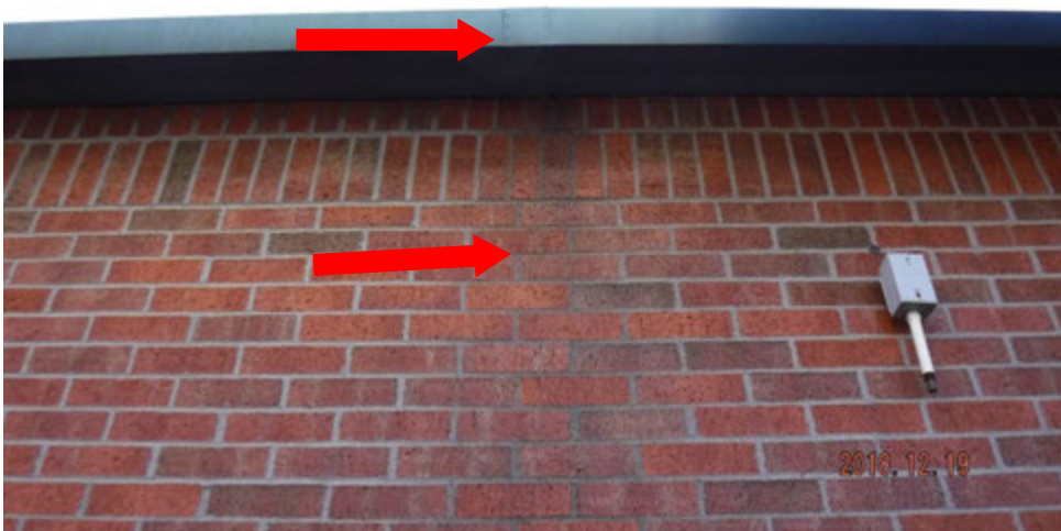
10b. Leaking gutter joint causing staining on masonry (see #10 on elevation photo for typical locations).
