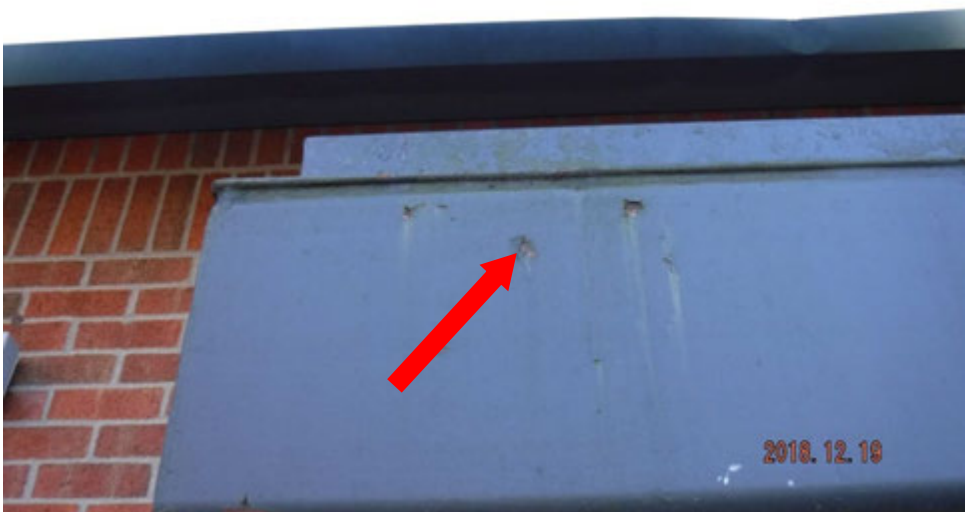
9b. Corrosion at canopy fascia (see #9 on elevation photo for location).
