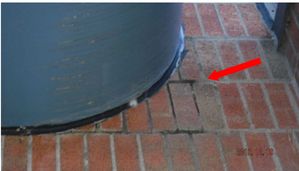
2b. Masonry appears to be holding moisture and not drying out as needed (see #2 on elevation photo for location).
