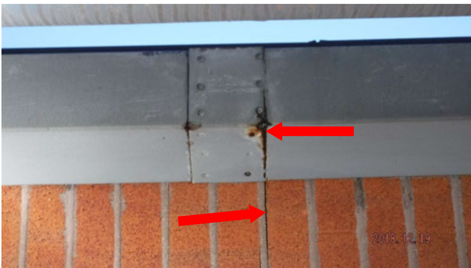
10a. Leaking gutter joint. The gutter is showing corrosion and water migrating down wall is causing masonry issues as well (see #10 on elevation photo for typical locations).
