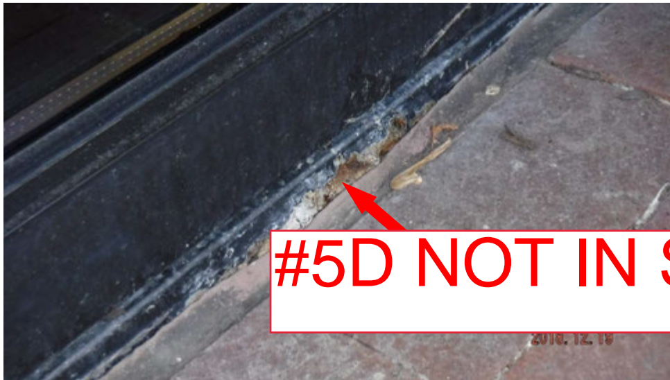
5d. Corroded steel member at base of window where it sets at ground level (see #5 on elevation photo for location).
