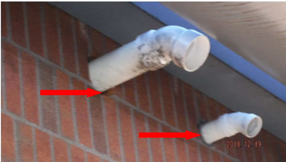
2b. Poor and/or missing sealant joints (see #2 on elevation photo for typical location).
