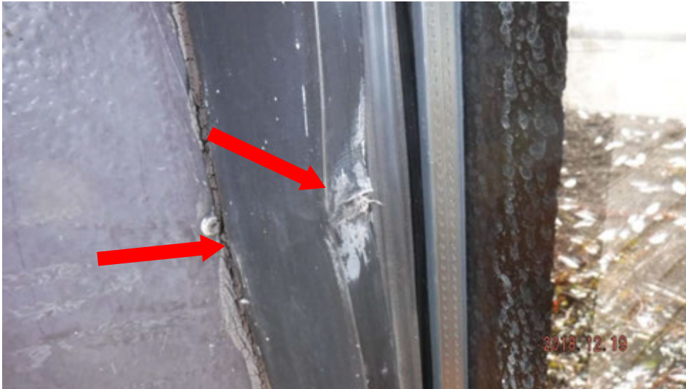
9b. Cracked/shrunk sealant joint and damage to window frame/pressure plate (see #9 on elevation photo for location).
