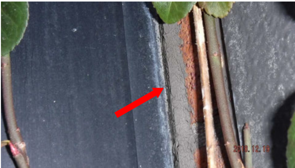
4b. Cracked/shrunk sealant joint (see #4 on elevation photo for typical locations).
