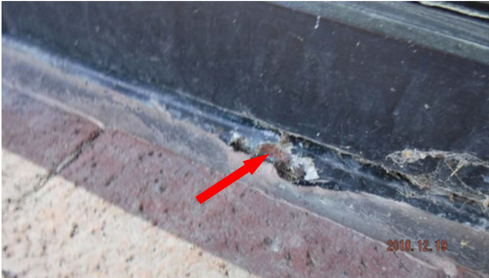
5b. Corroded steel member(s) at base of window where it sets at ground level (see #5 on elevation photo for location).
