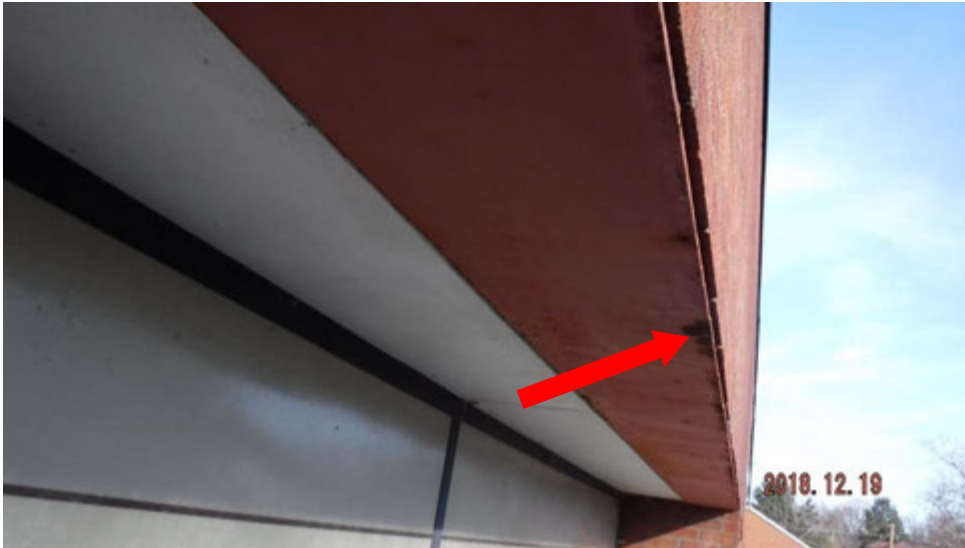
11c. Corrosion on window lintel (see #11 on elevation photo for typical locations).
