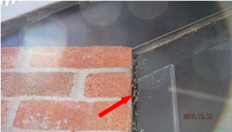
4b. Open joint between masonry wall and window frame (see #4 on elevation photo for location).
