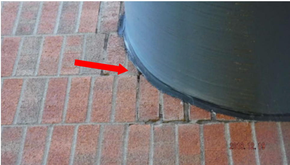
2a. Deteriorated mortar joints (see #2 on elevation photo for location).
