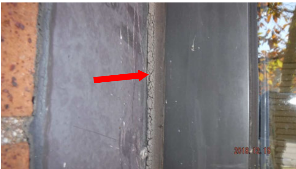
9a. Cracked/shrunk sealant joint (see #9 on elevation photo for location).
