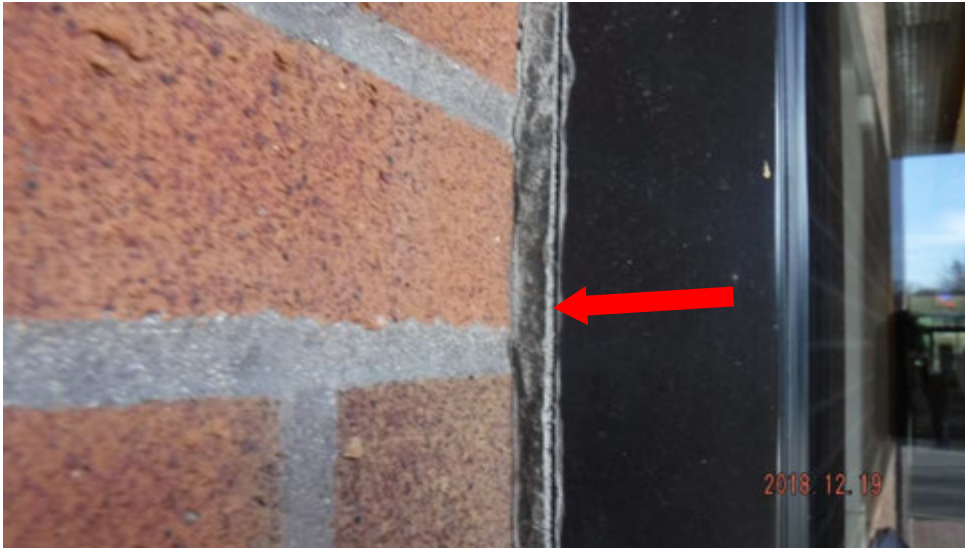
6c. Cracked/shrunken sealant joint (see #6 on elevation photo for typical locations).
