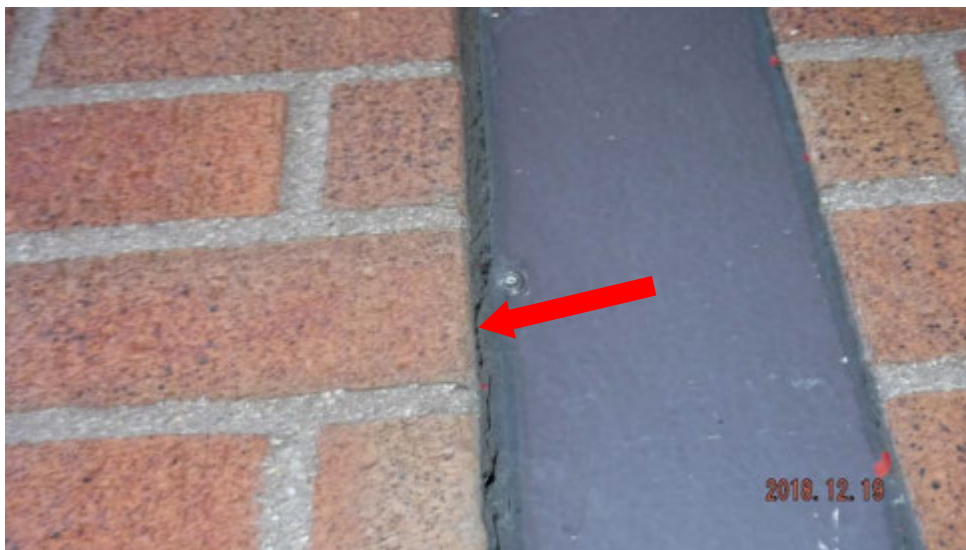
6a. Cracked/shrunk sealant joint (see #6 on elevation photo for location).
