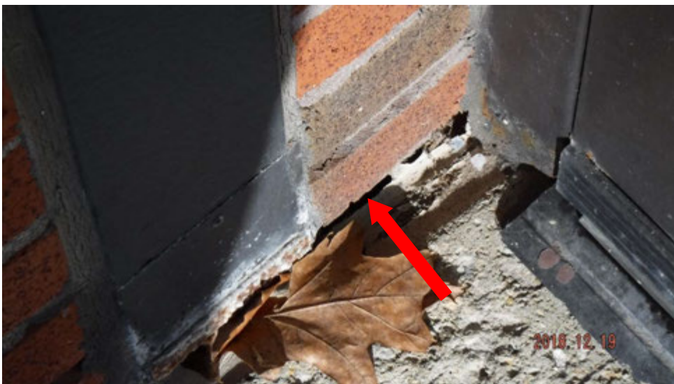
4a. Cracked/shrunk sealant joint between masonry wall and concrete sidewalk (see #4 on elevation photo for location).
