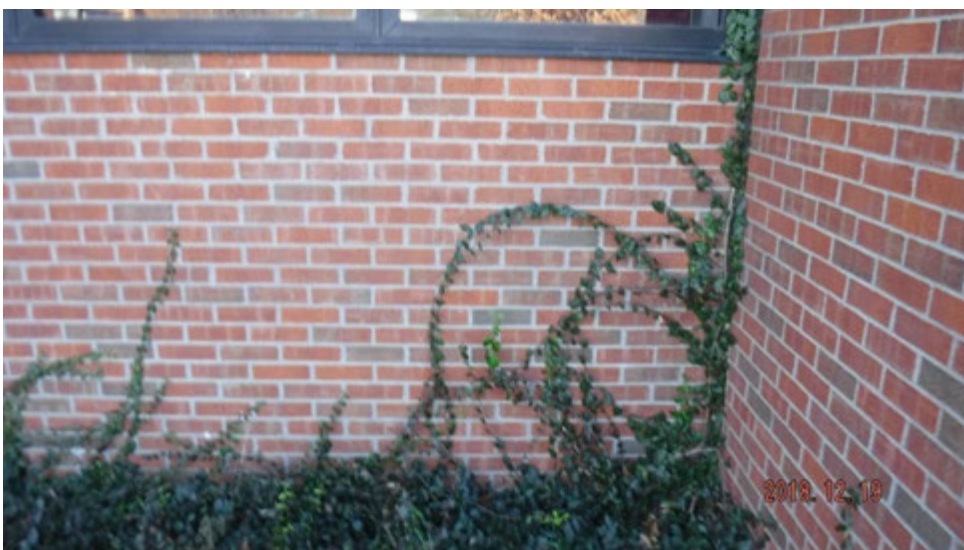
3a. Vegetation growth on walls (see #3 on elevation photo for typical location).
