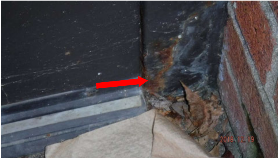
8a. Corrosion at door frame (see #8 on elevation photo for location).
