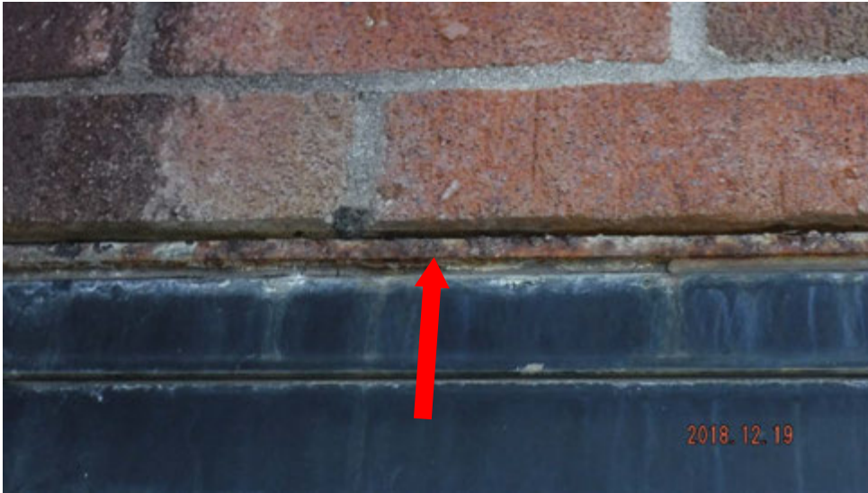
6a. Corrosion on window lintel (see #6 on elevation photo for typical locations).
