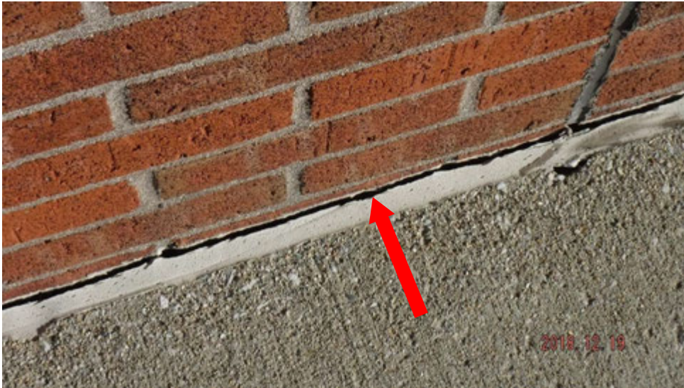
4b. Cracked/shrunken sealant joint between masonry wall and concrete sidewalk (see #4 on elevation photo for location).
