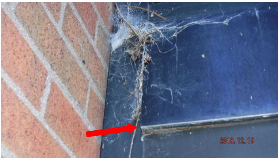
8b. Loose window trim metal between window sets. Wood could be observed behind the loose metal (see #8 on elevation photo for location).
