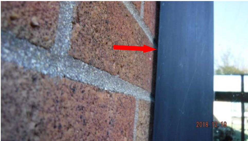
5a. Open joint between masonry wall and window frame (see #5 on elevation photo for location).
