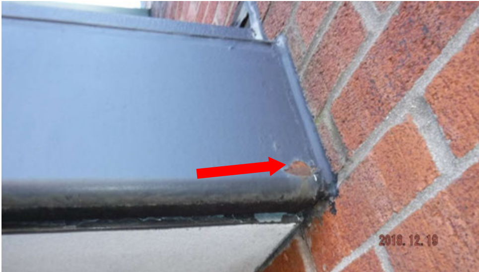
9a. Corrosion at canopy fascia (see #9 on elevation photo for location).
