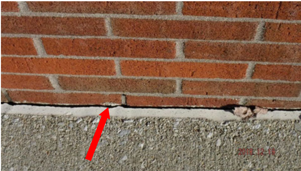
4c. Cracked/shrunken sealant joint between masonry wall and concrete sidewalk (see #4 on elevation photo for location).
