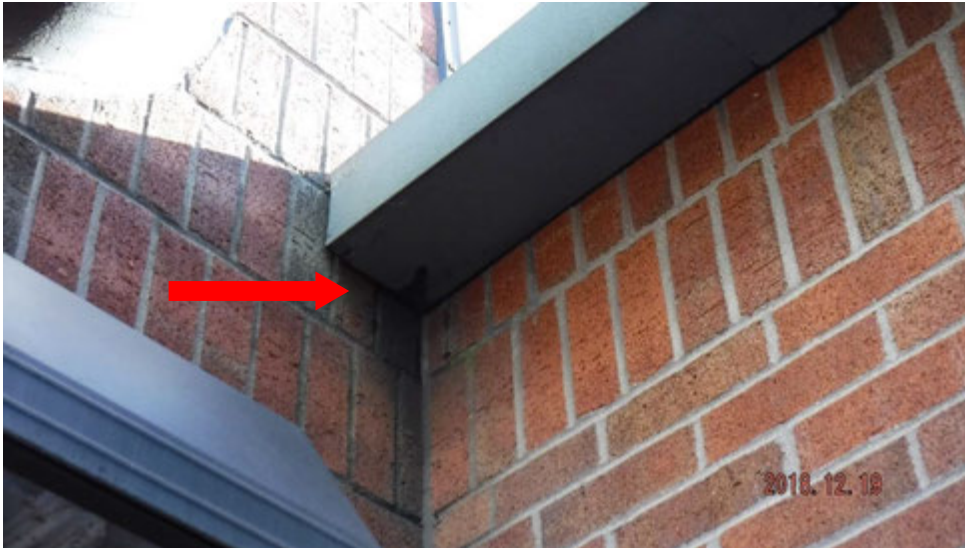
10c. Leaking gutter end cap (see #10 on elevation photo for typical locations).
