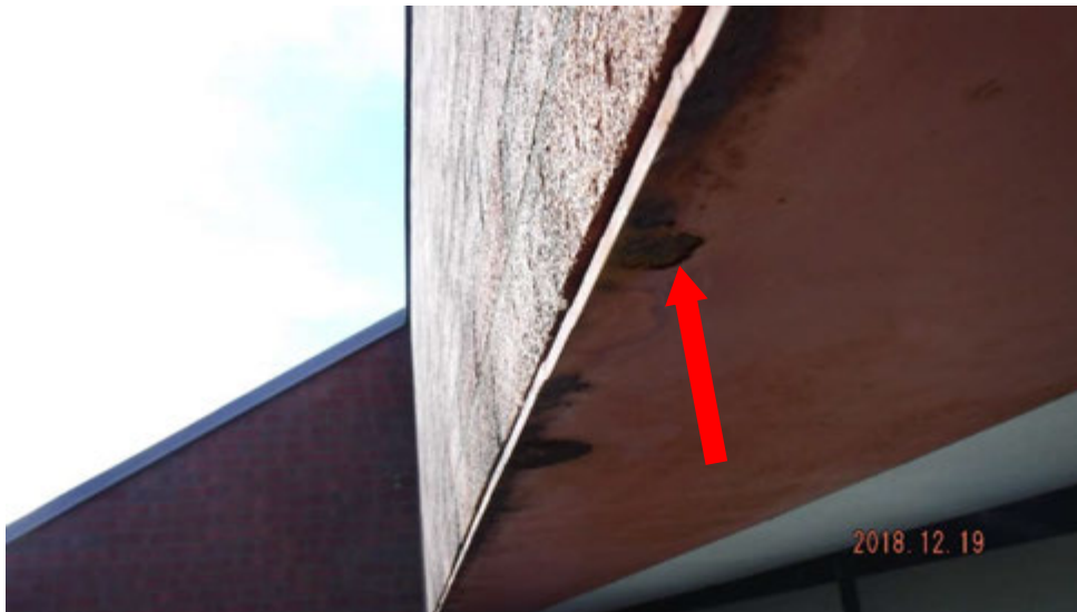
11b. Corrosion on window lintel (see #11 on elevation photo for typical locations).
