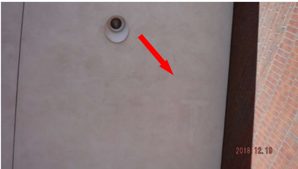
4a. Crack in plaster ceiling (see #4 on elevation photo for location). Hard to see in picture but is there.
