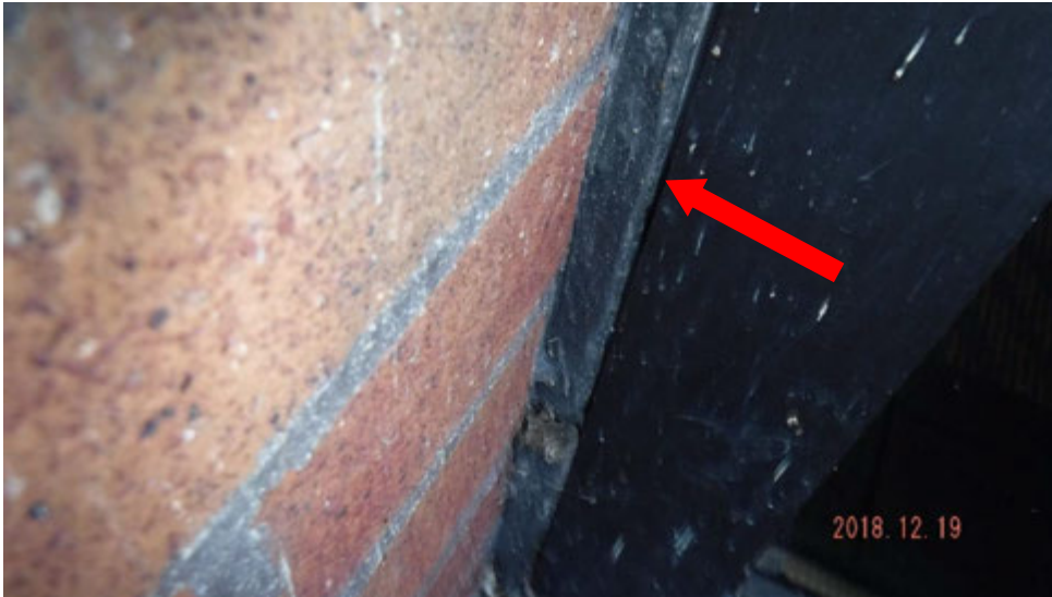
6b. Cracked/shrunk sealant joint (see #6 on elevation photo for typical locations).
