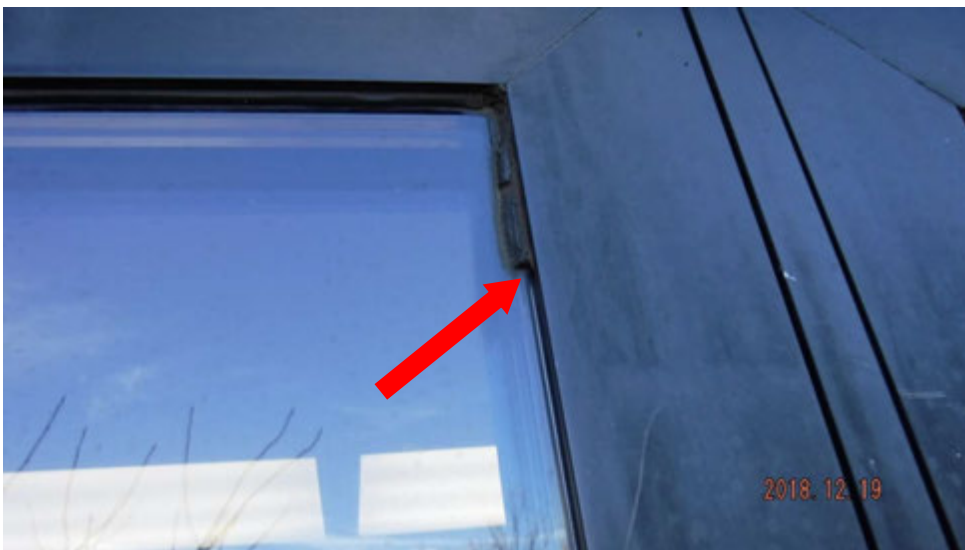
5b. Deteriorated and/or missing sealant between window glass and frame (see #5 on elevation photo for location).
