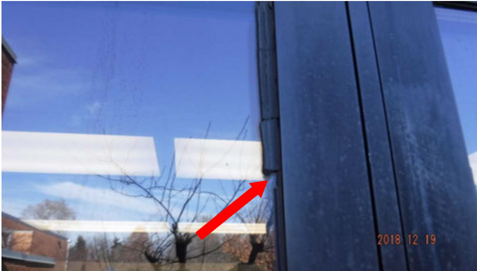
5a. Deteriorated and/or missing sealant between window glass and frame (see #5 on elevation photo for location).
