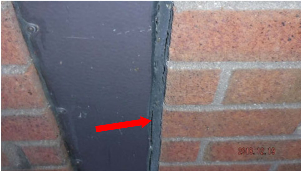
6b. Cracked/shrunk sealant joint (see #6 on elevation photo for location).
