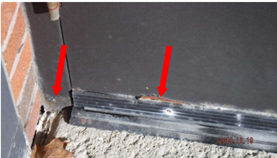
7b. Corrosion at door and door frame (see #7 on elevation photo for location).
