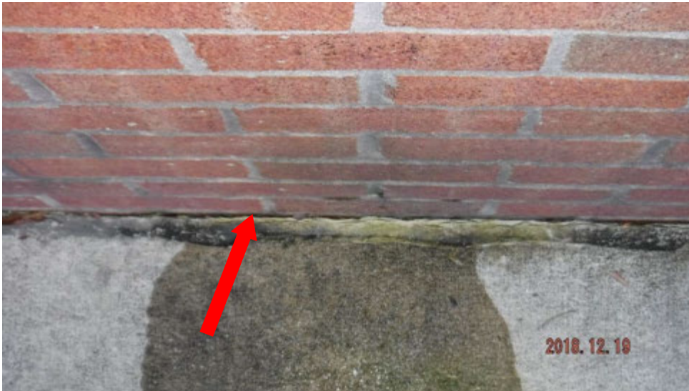
2a. Cracked/shrunk sealant joint between masonry wall and concrete sidewalk (see #2 on elevation photo for location).
