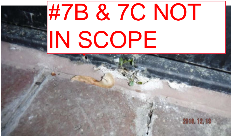
7c. Corroded steel member(s) at base of window where it sets at ground level (see #7 on elevation photo for location).
