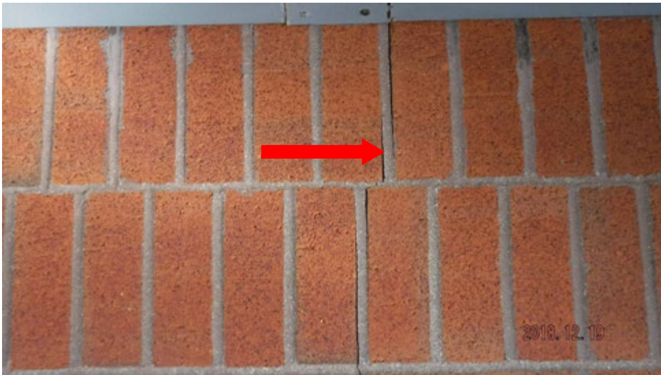
1a. Cracked/shrunk mortar joints (see #1 on elevation photo for location).
