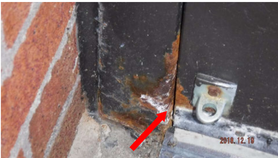
8b. Corrosion at door and door frame (see #8 on elevation photo for location).
