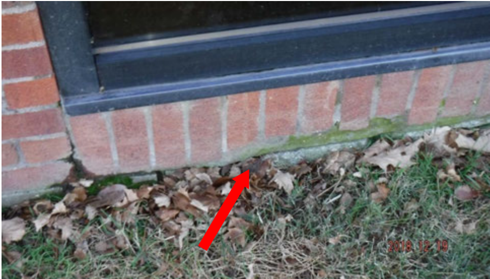
1a. Poor/deficient foundation below window (see #1 on elevation photo for location).
