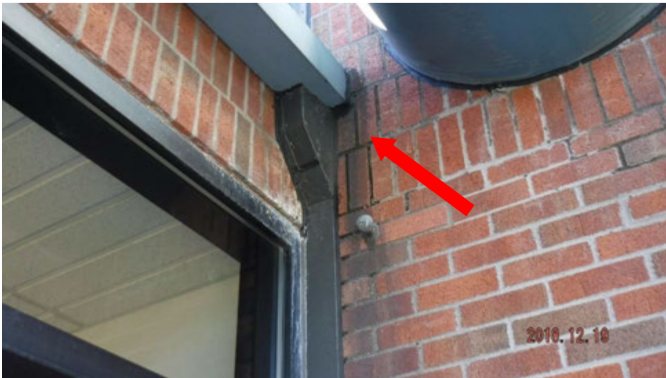
10d. Leaking gutter end cap and/or connection to downspout (see #10 on elevation photo for typical locations).
