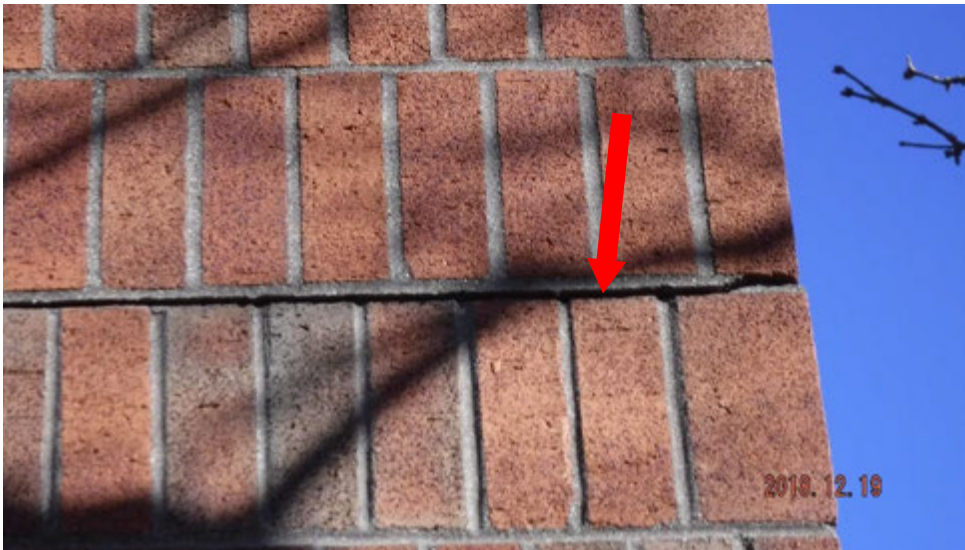
1a. Cracked/shrunk mortar joint (see #1 on elevation photo for location).
