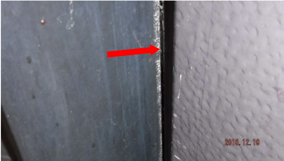
9f. Cracked/shrunk sealant joint (see #9 on elevation photo for location).
