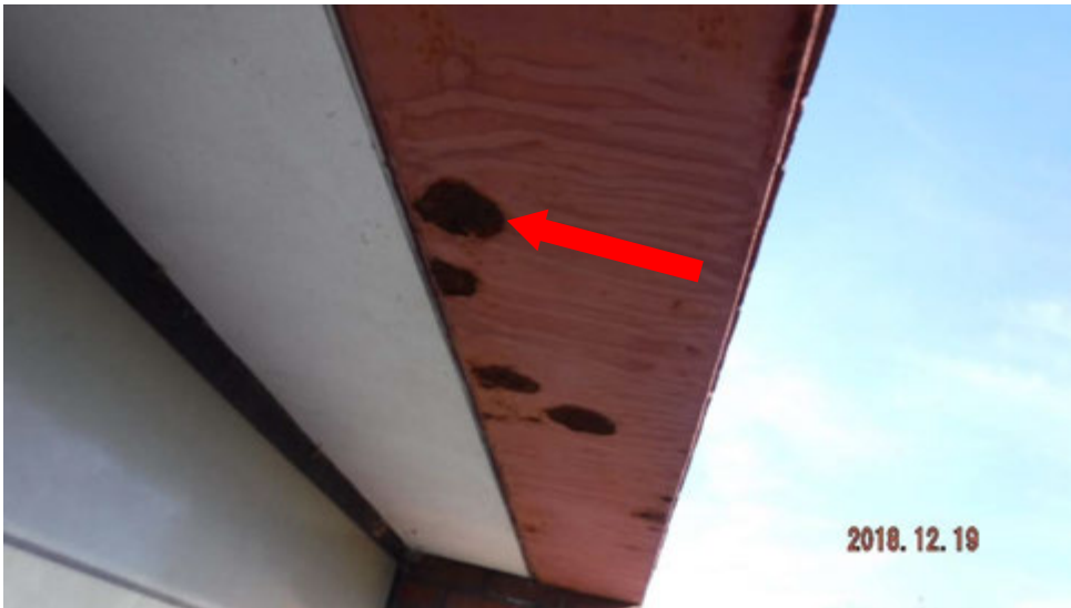
11d. Corrosion on window lintel (see #11 on elevation photo for typical locations).
