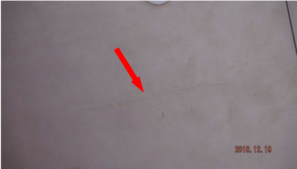
4b. Crack in plaster ceiling (see #4 on elevation photo for location).
