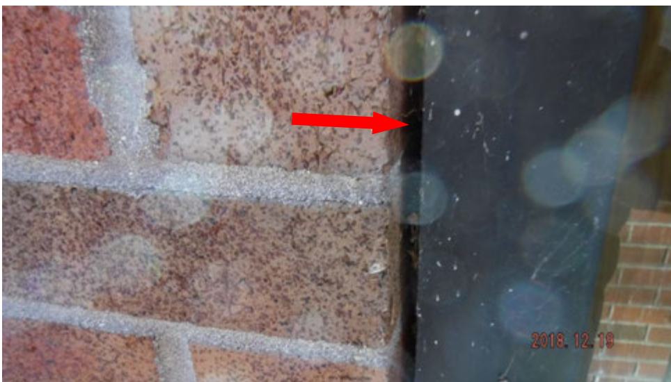
4a. Open joint between masonry wall and window frame (see #4 on elevation photo for location).
