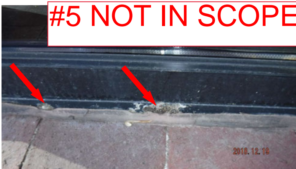
5a. Corroded steel member(s) at base of window where it sets at ground level (see #5 on elevation photo for location).
