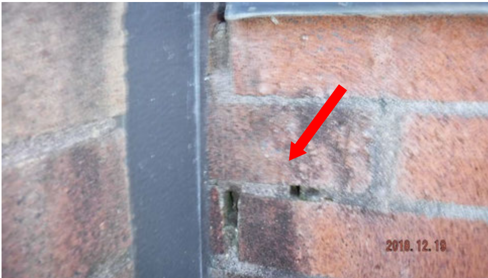
1a. Deteriorated mortar joints (see #1 on elevation photo for location).
