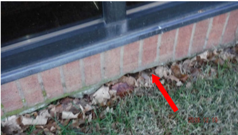
1b. Poor/deficient foundation below window (see #1 on elevation photo for location).
