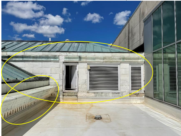
South facing vertical marble panels and top side of horizontal cornice capstone ledges
